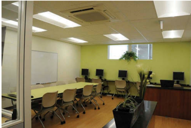
Figure 5. Updated LED lighting and air conditioning system.
